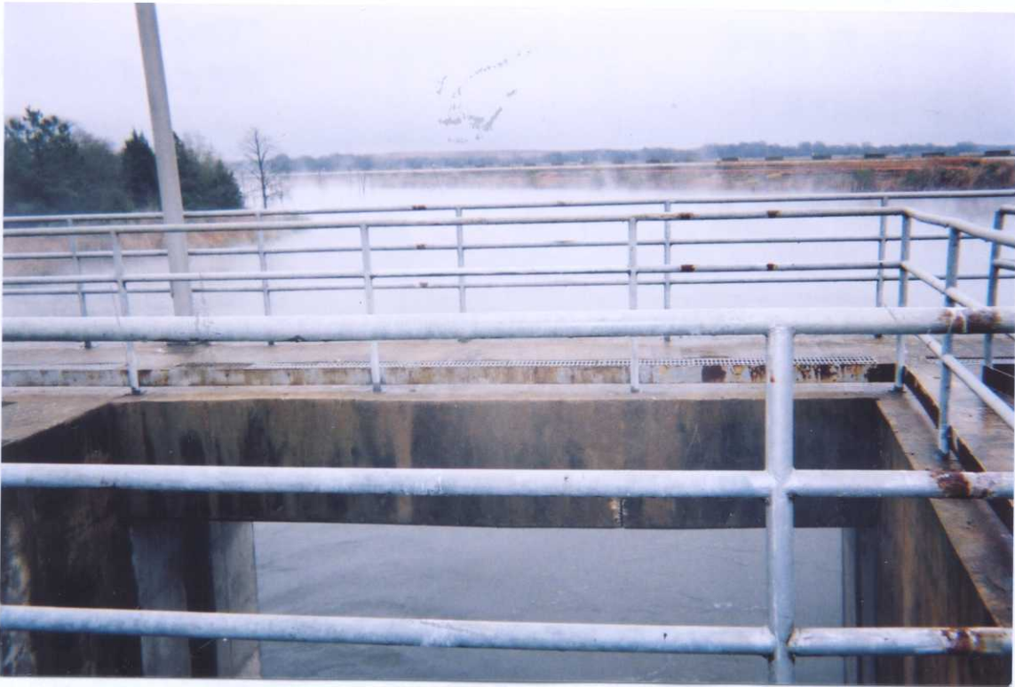
Outfall 004 Texas Municipal Power Agency Gibbons Creek Steam Electric Station Carlos, Texas
