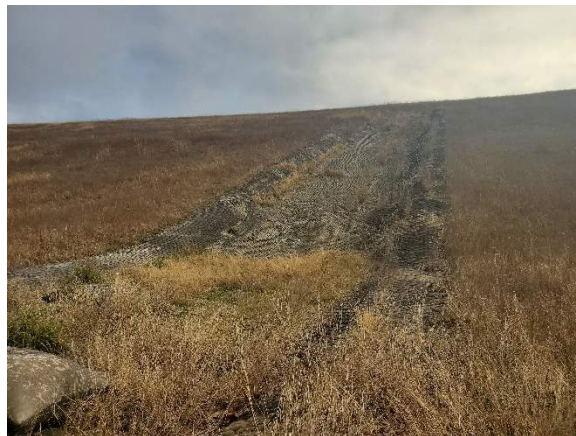
Figure 5: Vegetation and Sediment on Concrete Revetment
