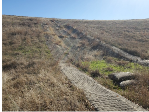
Figure 5: Vegetation and Sediment on Concrete Revetment
