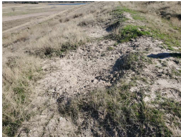
Figure 4: Side Slope Erosion
